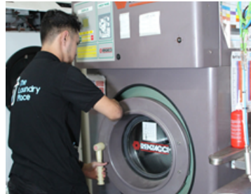
DRY CLEANING MACHINE - RENZACCI UK 3 X 23KG MACHINES 3,000 PIECES/DAY
